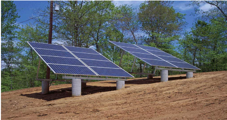
Fig. 2. Ground mounted solar PV
