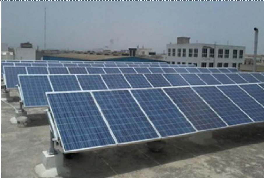
Fig. 3. Roof top solar power PV plant
